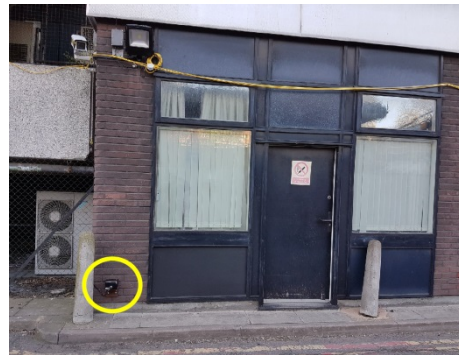
MRI Scanner Room 4
